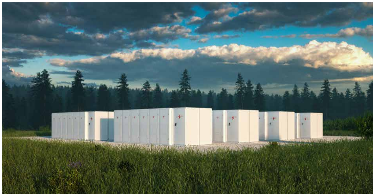
Figure 6.11-1: Utility Scale Battery Storage Example 62
