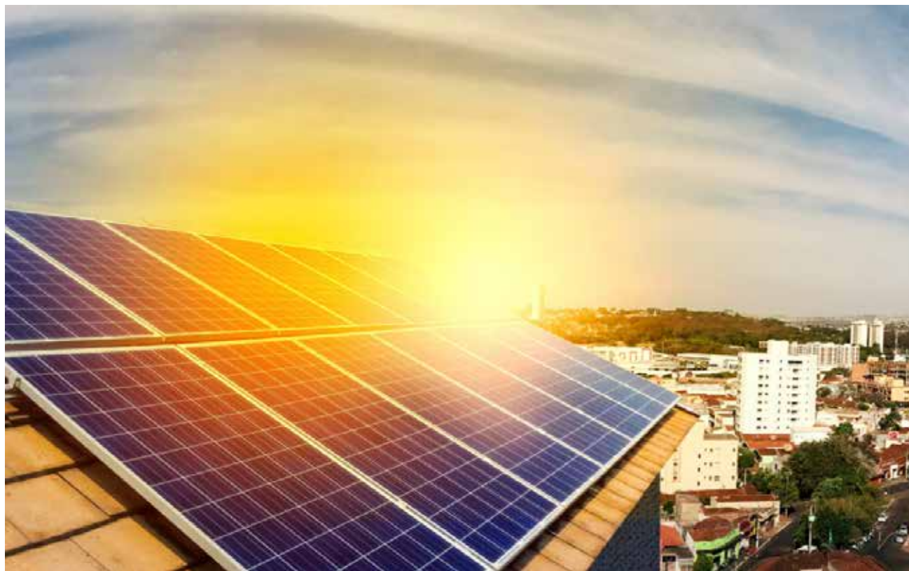
Figure 6.13-1: Rooftop Solar Panel 72
